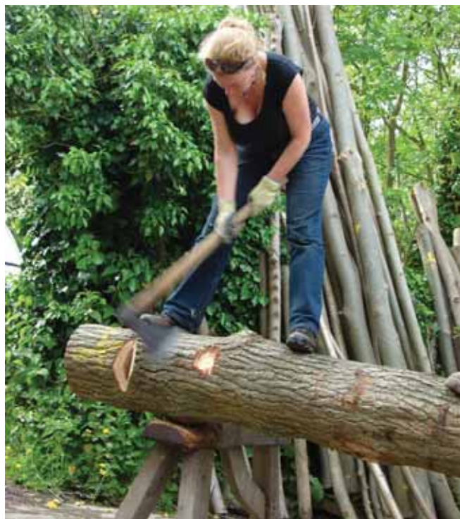
Hewing a log into a sole plate for use in the repair programme
