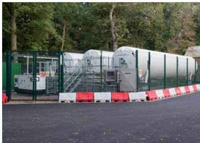
Liquid CO 2 is stored in large tanks by the main buildings
